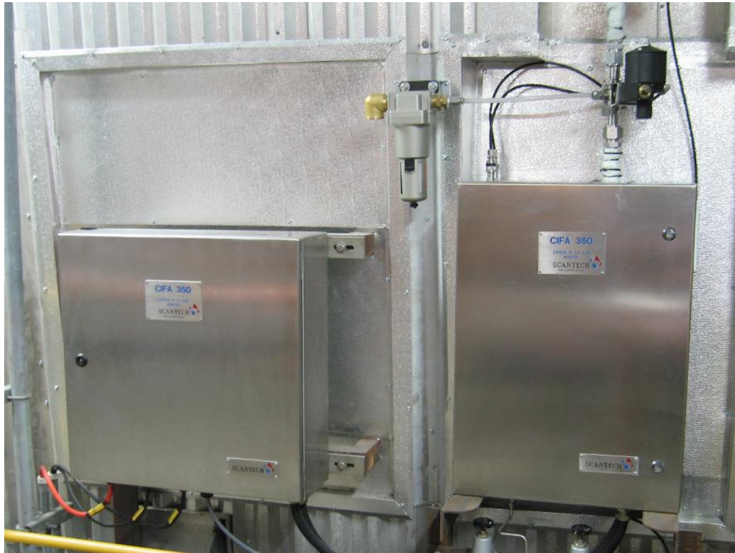
Figure 1. - CIFA350 Electronics Module and Measurement Module on a Duct
